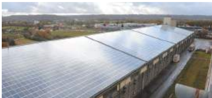
Photovoltaic roof of the Aire-sur-l'Adour site
